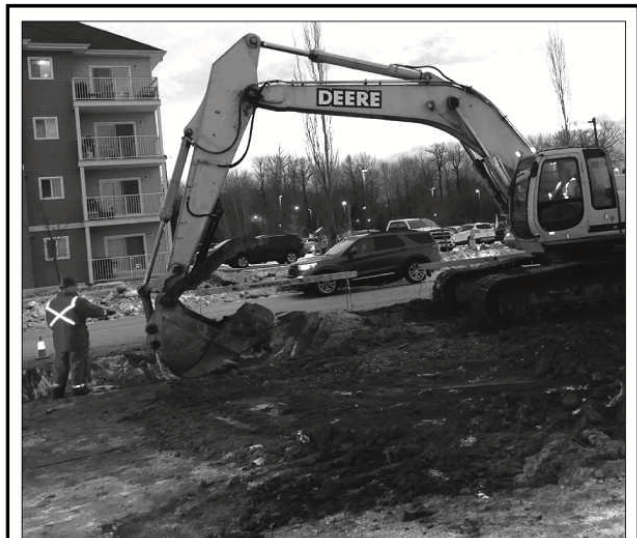
The water line repair at 6th Ave. and 6th St. SE on Jan. 23 wasn't the only one; the Town of Slave Lake did another one last week on 11th Ave. SE. The one pictured was on a main line. It had been discovered a couple of days earlier. "It cracked right in half," says TOSL Director of Operations Calvin Couturier. A few days later, the town was back at it, digging up the leaking line on 11th Ave.
